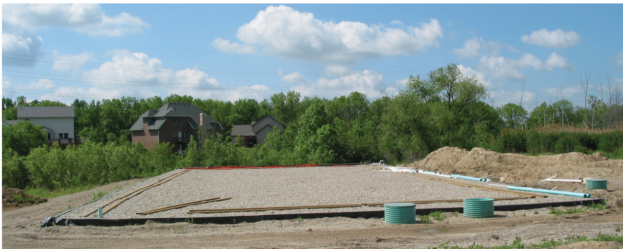
Recirculating Media Filter
